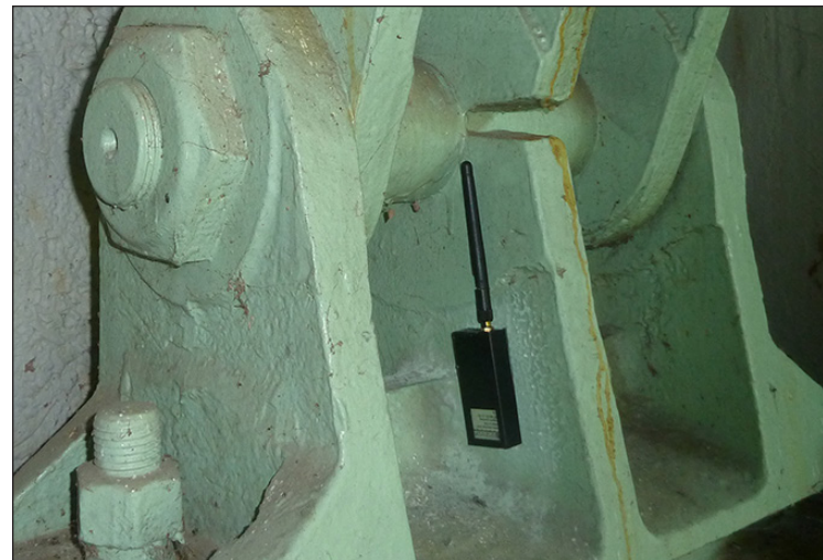
Figure 4. Resensys structural stress sensors mounted beneath bridge trusses require extended life bobbin-type \text{LiSOCl}_2 batteries to reduce the need for costly and dangerous work to replace batteries in such hard-to-access locations.
